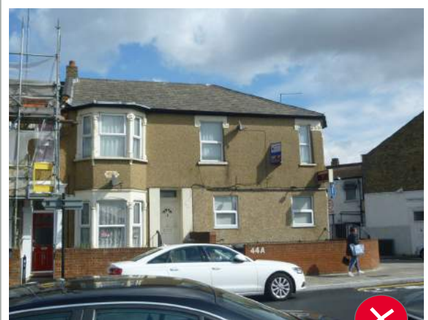
Brickwork should not be painted or covered with render, pebble-dash or cladding.
